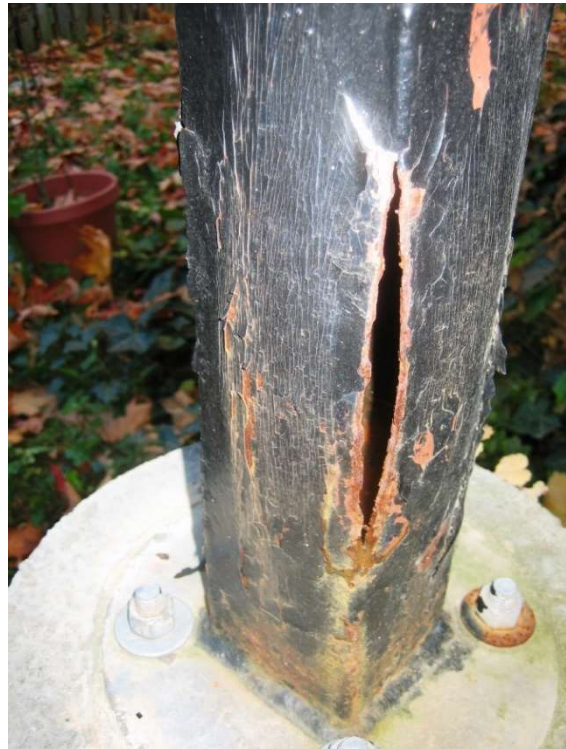
Corrosion of steel post base
