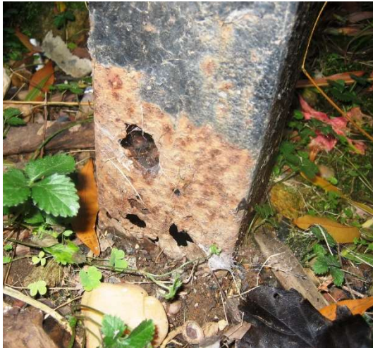
Corrosion of steel post base
